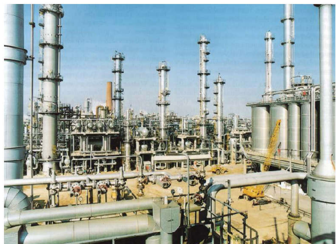
Figure: Ethylene plant (ROW Wesseling)
