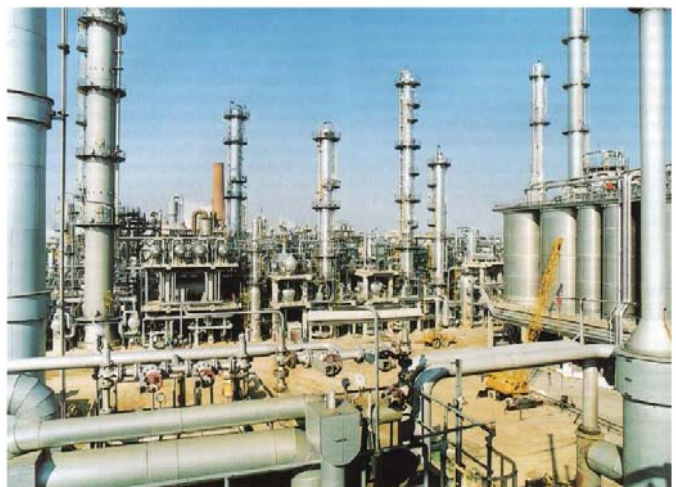
Figure: Ethylene plant (ROW Wesseling)
