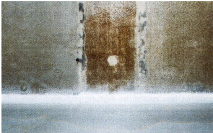
Biofilm formation on concrete wall of a water storage tank (Herb et al., 1999)
