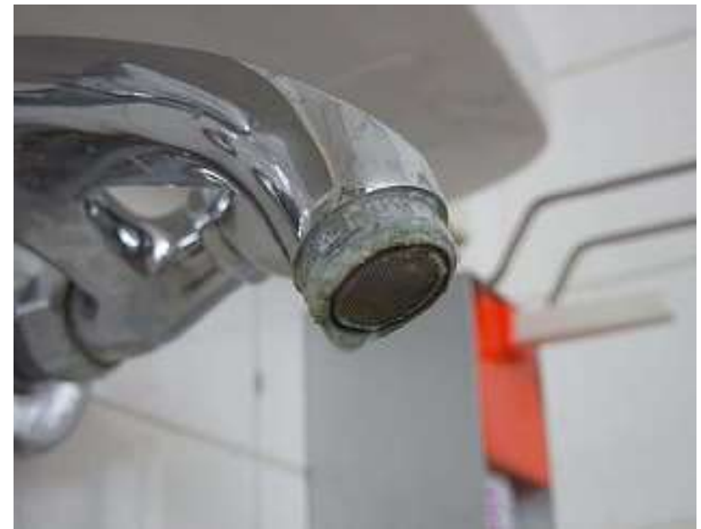
Biofilm on corroded faucet flow straightener.
